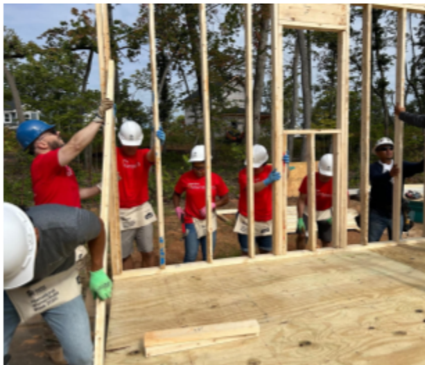
Wells Fargo employees (in red) along with a future Habitat homeowner (Omar Montelongo, in gray) erect the first wall of a shed built for scratch that will accompany one of the new homes in Dixon Village.
