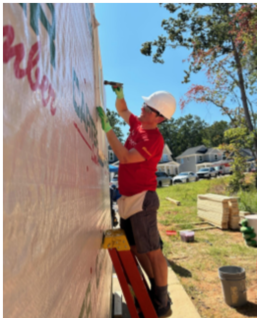
A Wells Fargo volunteer nails a window frame to a newly constructed shed.
